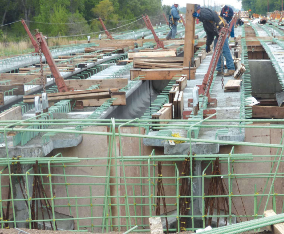
NU 1100+25 prestressed concrete girders are in place, and reinforcement is being placed for the abutment. Bent strands extending from girders are used for the connection to the abutment as well as in diaphragms between spans.
