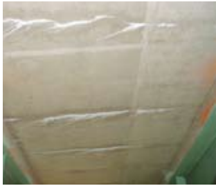
Transverse cracking on underside of Bridge No. 2668N.
