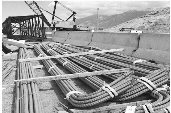
Store bars above ground on protective cribbing
