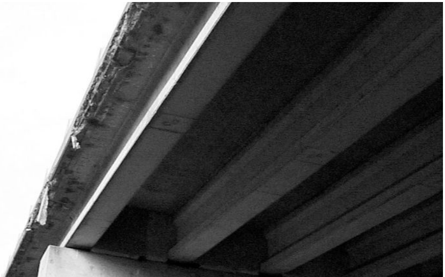
Corrosion damage to underside of deck constructed with uncoated reinforcement
