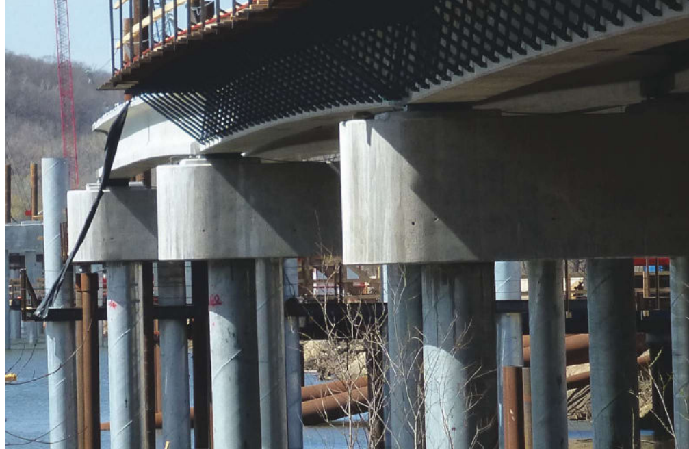
The bridge was constructed in multiple segments. The spiral welds are visible on the steel pipe piles that were filled with concrete after driving.
