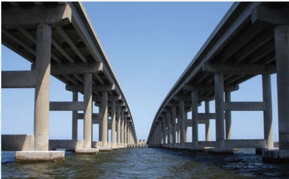
Figure 4: Companion bridges containing either black (left) or epoxy-coated bars (right) in Melbourne Florida.
