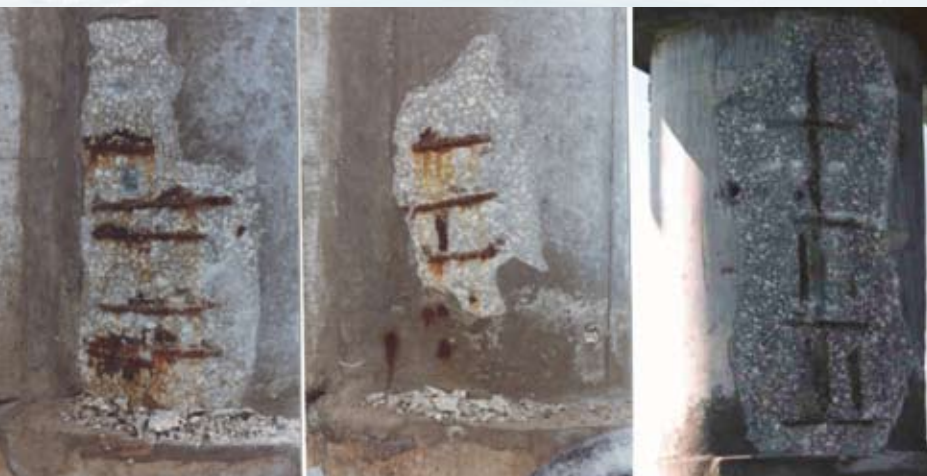
Figure 1: Typical spalls observed in bridge piers (1) .
