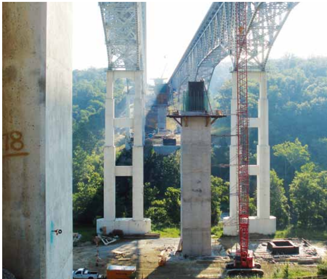
Each of the twin structures consists of a single cell, variable depth box girder. Photo courtesy of James E. Barnhart, Ohio Ready Mixed Concrete Association.
