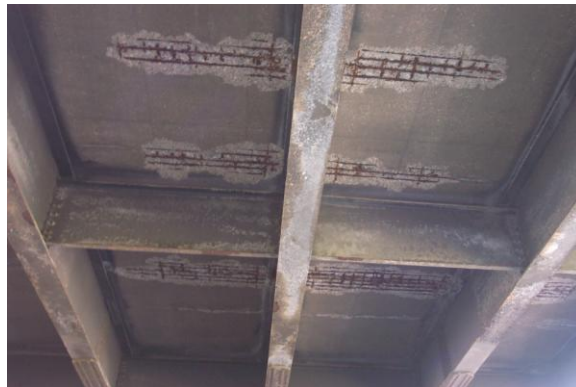
Figure 6: Deterioration of bridge deck using uncoated bars as bottom mat and epoxy-coated bars as the top mat
