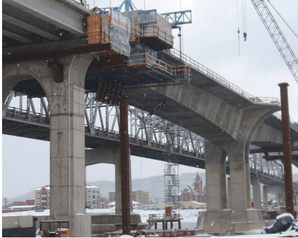
Form travelers with suspended heated enclosures enabled concrete for the segments to be placed throughout the winter. Photo: FIGG.
