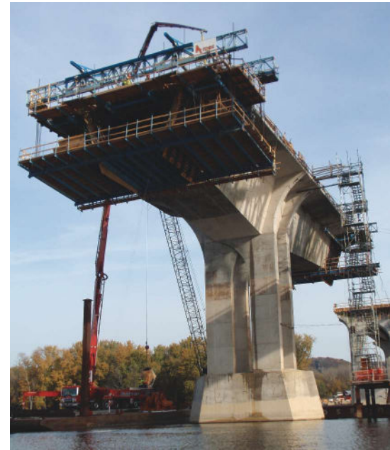
The main river spans utilized the cast-in-place balanced cantilever construction method. Photo: Minnesota Department of Transportation.
