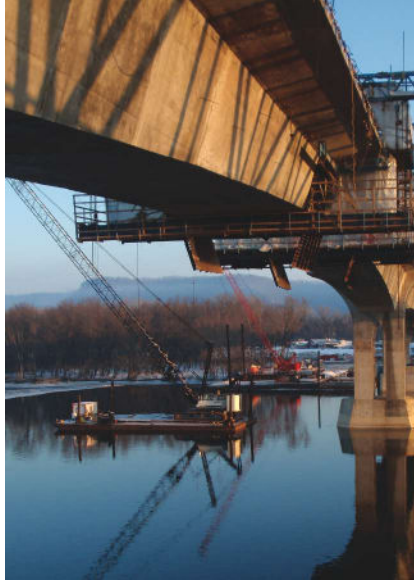
The segmental box girder, which mirrored the historic cantilever through-truss, gained acceptance and was also the most cost-effective alternative. Photo: FIGG.
