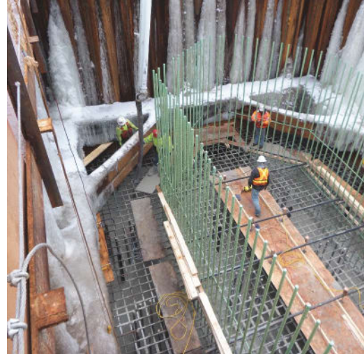
An early foundations contract was used to accelerate construction of the river pier foundations. Photo: Minnesota Department of Transportation.
