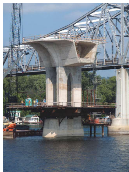
The pier table was constructed one-half segment out of balance with 28 ft projecting into the main span and 20 ft into the back span. Photo: FIGG.
