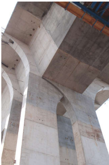
Main river piers are 3 ft by 9 ft 6 in. and extend 45 ft above the top of the ice breaker to the pier table. Photo: FIGG.
