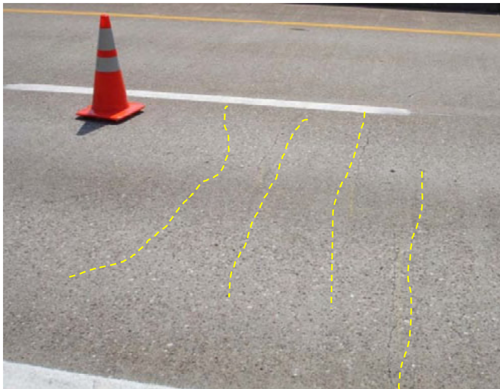
Figure 14. Transverse cracking in Bridge No. 2672S. Cracks are highlighted by yellow dashed lines.
