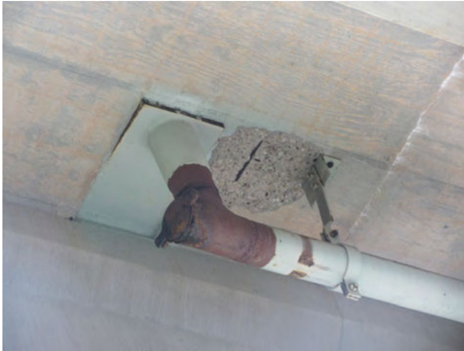
Figure 16. Spall due to corrosion of uncoated bottom bar in Bridge No. 2672N.
