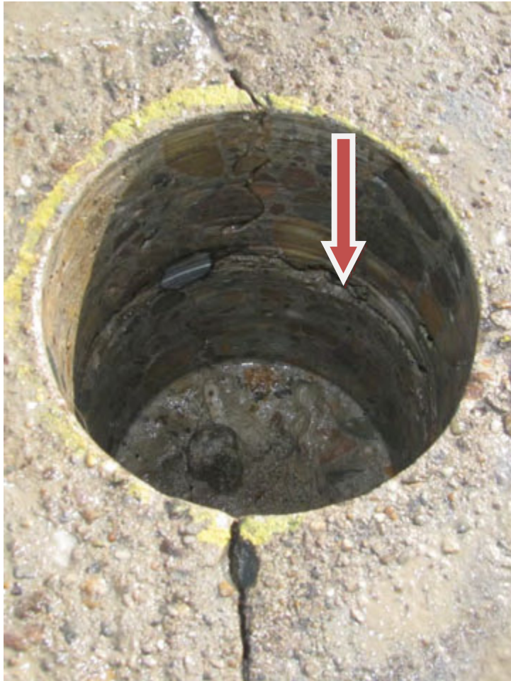
Figure 25. Delamination at bar level caused by corrosion of uncoated black bar in Bridge No. 2930.
