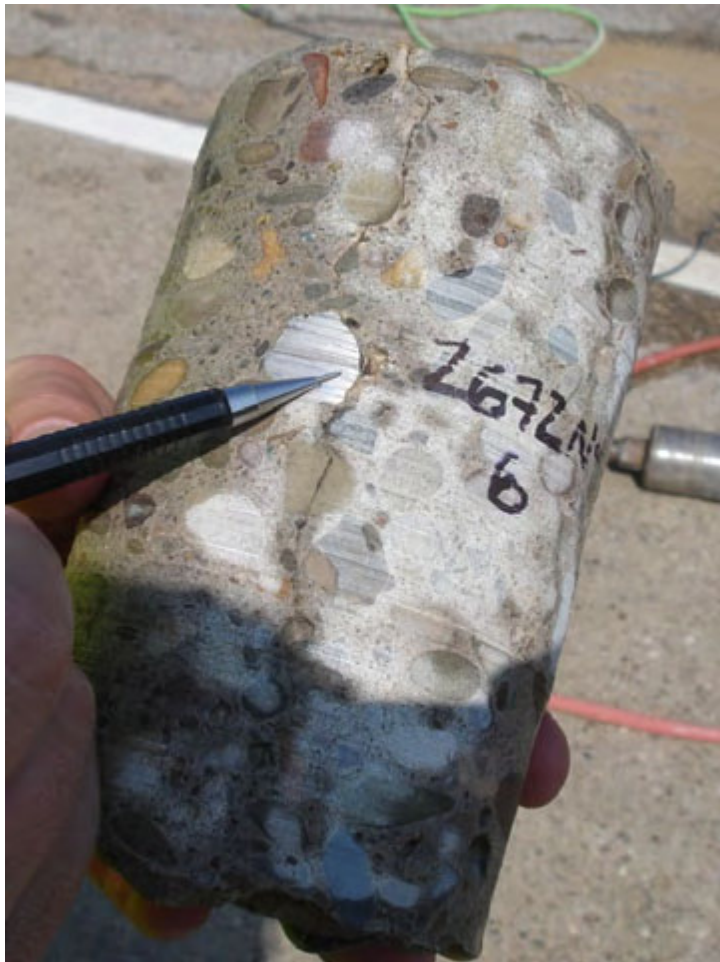
Figure 15. Transverse cracking core 6 from Bridge No. 2672N.
