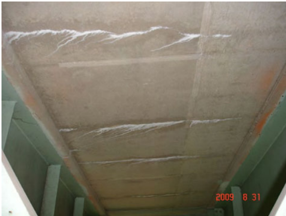
Figure 10. Transverse cracking on underside of Bridge No. 2668N.
