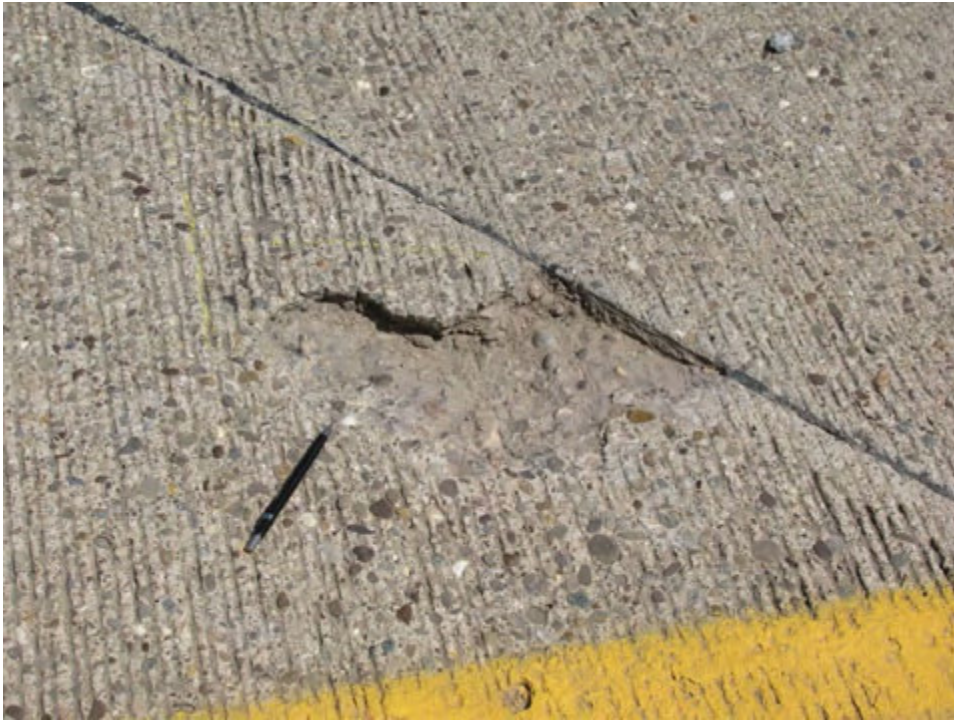
Figure 18. Spall at construction joint on Bridge No. 2673.
