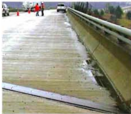
Small percentage of damage at railing barriers caused by corroded bars.
