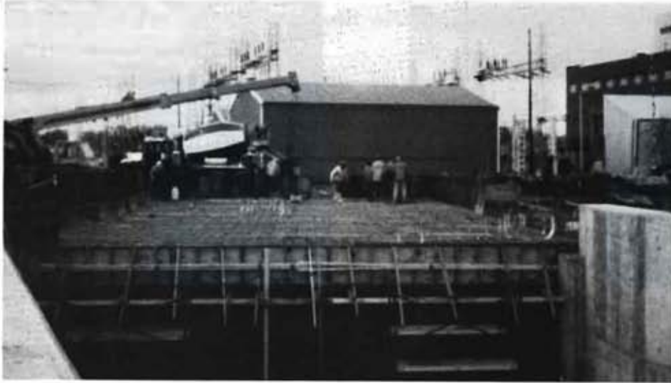
Pouring the deck over the water treatment plant. All rebar is epoxy-coated.
