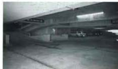
Street level of the garage. Grade 60 epoxy-coated steel was specified for the parking ramps, and decks on all seven of the parking levels.
