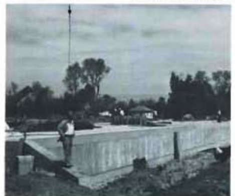
Flume was built on grade to facilitate construction and excavated for I-70 to pass beneath it.
