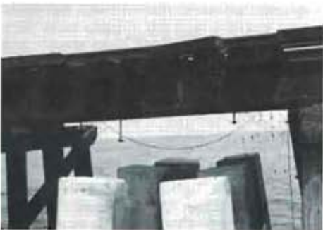
The six pile concrete bent and steel bent in place ready to receive poured-in-place concrete cap.
