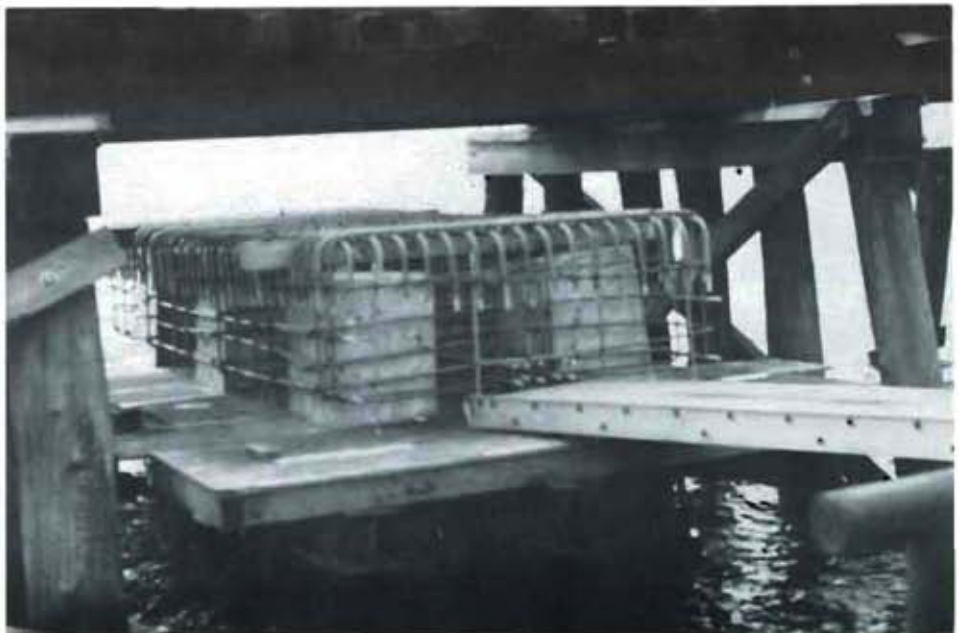
Rebar cage of Grade 60 epoxy-coated steel in place ready for forming and pouring.
