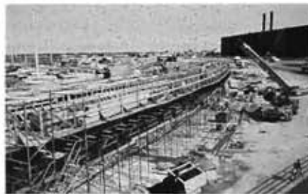
After passing Terminal 4, the new extension splits off from the existing roadway to descend to grade for the trip out of the airport.
