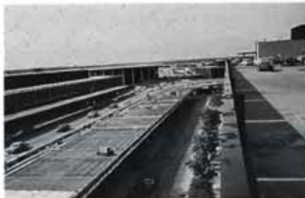
Passing Terminal 3, installation of the epoxy-coated rebar is nearly complete; ready for deck construction.
