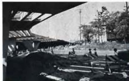
The widely spaced and graceful piers with cantilevered roadway make an attractive addition to O'Hare's transportation facilities.
