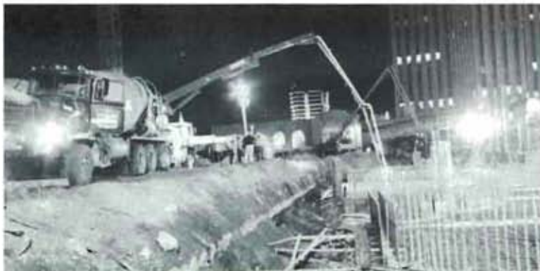
Construction gets underway with the placement of concrete for the mat foundation.
