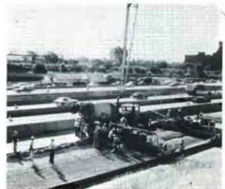
View of the paving on one of the ramps where the contractor used a pump to place some of the concrete at this location.
