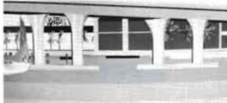
(Photo Top Left) Construction of the Pier foundation (within Biscayne Bay) proceeds with epoxy-coated reinforcing steel. The original bridge with railroad trestle is beside the new structure.
