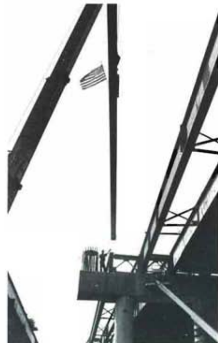
The final beam, adorned with an American flag, was placed on August 8 this year. The entire project, reconstruction of the south and northbound lanes, enlarged from 8 to 10 lanes, was completed ahead of schedule; earning the contractors substantial bonuses.
