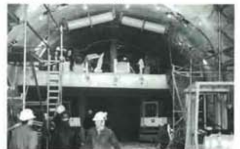
Looking into tunnel as first section is jacked slowly in place while excavation goes on.
