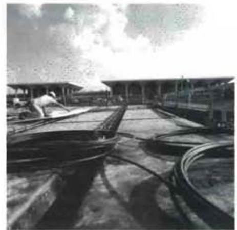
Installing epoxy-coated rebar on the new third level of the enlarged parking facility.
